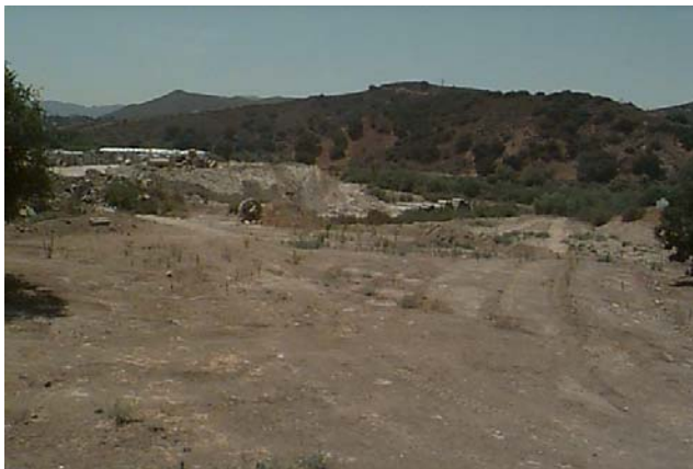
b. View from Los Angeles Ave. of restoration site with Southdown Concrete Products facility on left.
