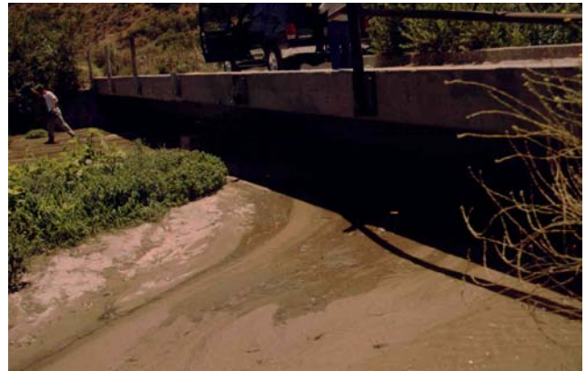
d. Bridge with only 15 inches of freeboard near Somis
