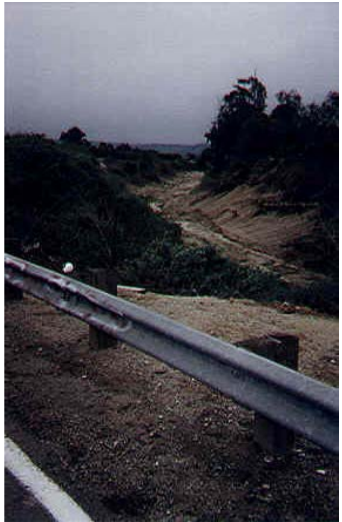
Site 10. Fox Barranca at Barylwood Road, down-gradient.
